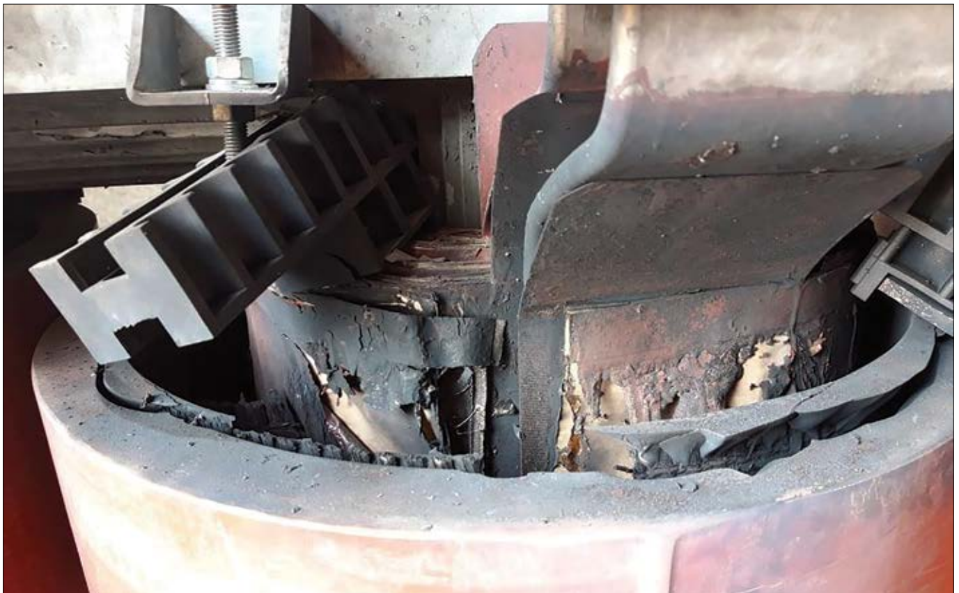
Fig. 4. The destructive effect of an electrical fault. Catastrophic discharge destroyed the central phase and charred part of the resin. The VOC sensor positioned above the phase was hit by the blow and failed.
