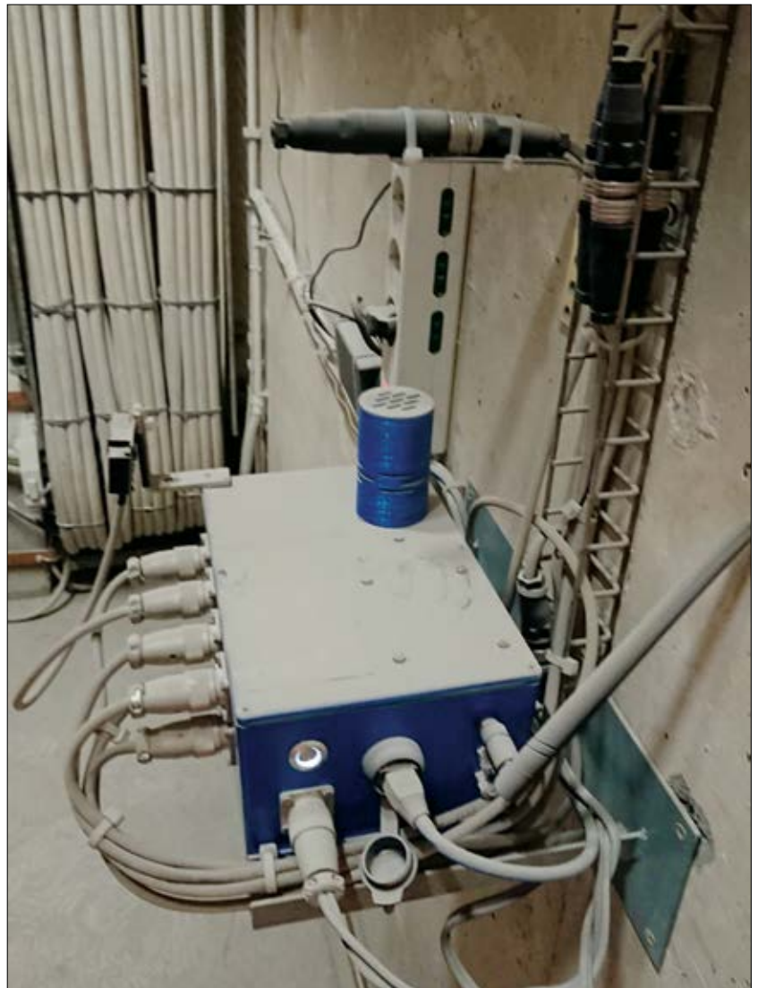
Fig. 11. Data acquisition device after a few months in a dirty room.
